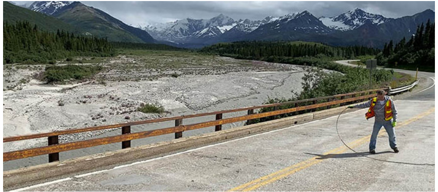
Bridge #581, Miller Ck., Richardson Highway. Statewide DES Bridge Section inspector Elmer Marx "Chain Drags" the bridge deck to locate concrete delaminations. By Hiram Henry, Alaska DOT&PF
